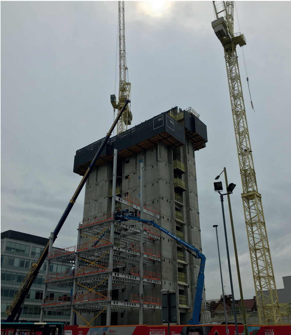
/ Site progress photo. The concrete core of the building has reached Level 10
